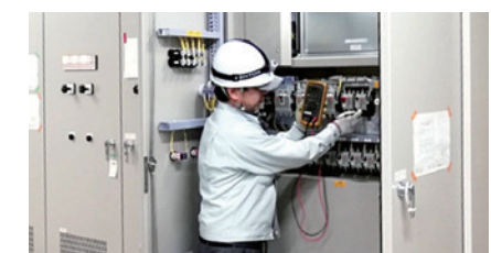
Maintenance and inspections by Sansha Solution Service
