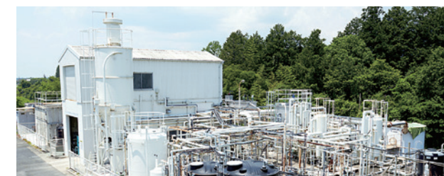
Wastewater treatment facilities at the Okayama Plant
