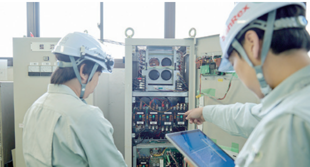
Power supply maintenance and inspection services
