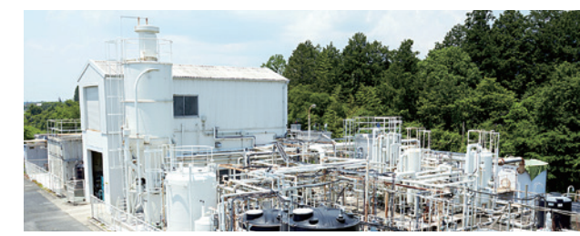
Wastewater treatment facilities at the Okayama Plant
