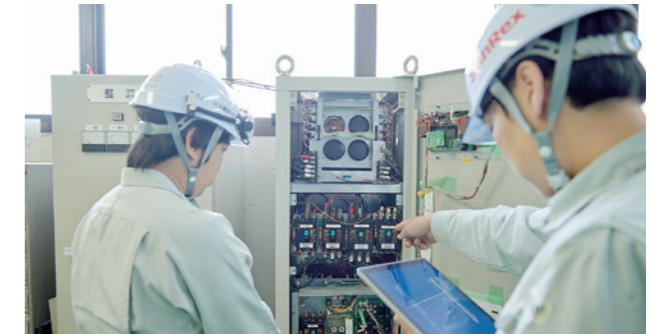
Power supply maintenance and inspection services
